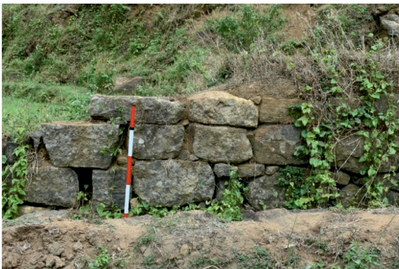
Photo 11: The way rock blocks have separated due to the removal of wedge stones
