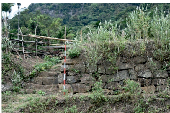
Photo 13. A location with a staircase to descend from a spot where a narrow terrace has been widened using rocks
