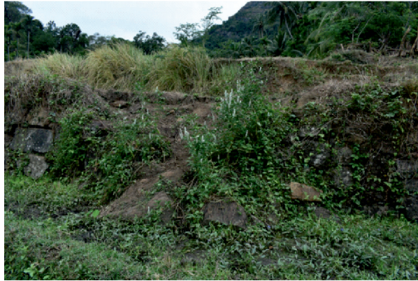
Photo 14: A location where a stone wall used to widen a narrow terrace has later collapsed
